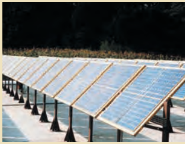
Photovoltaic panels for producing electricity.
