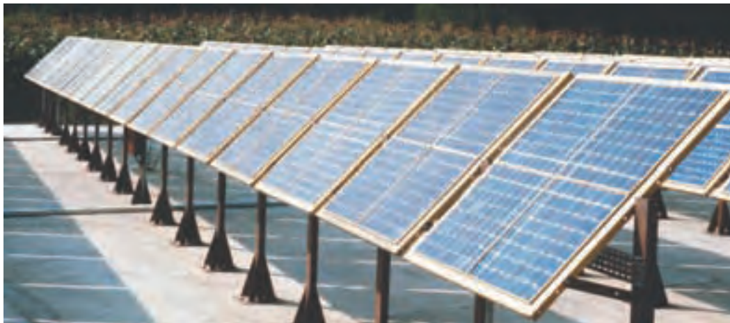
Energy savings requires the development of new energies.
